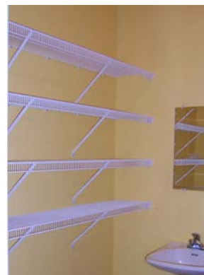
Noble Warriors helped coordinate installation of shelving at Commonwealth Clinic. Rearrangement of storage and other modifications will allow the clinic to better serve their dental patients.
